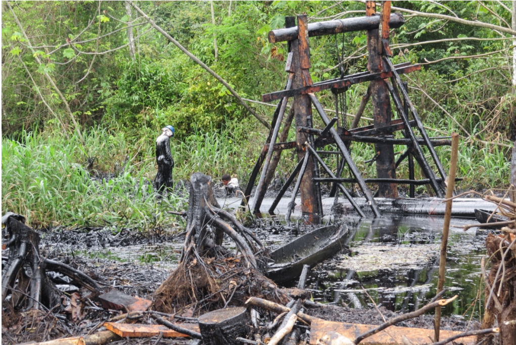
Photo 1: An indication of the pipeline's chronic state of disrepair and the impact that the Cuninico oil spill has had on the surrounding environment (Photo given to me by a Cuninico resident who himself received it from a Petroperu worker and used with their permission, June 2014).
